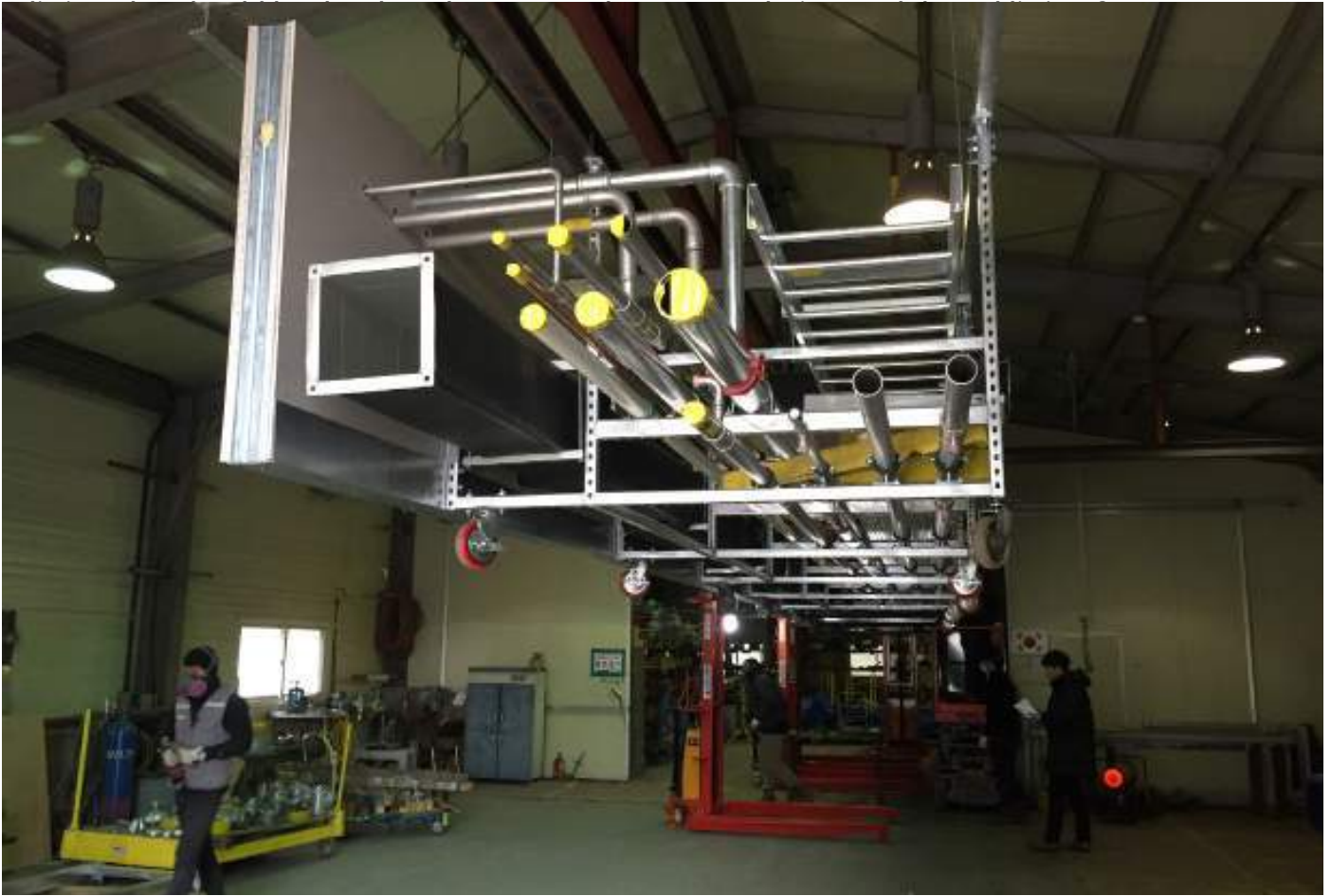
Figure 15: In Korea, prefabricated MEP modules are connected on the floor at the job site and lifted as a complete module for final installation. Synchronised wireless jacks are used to maintain alignment when lifting the module. (Photograph courtesy of Hyundai Engineering & Construction Pte Ltd)
