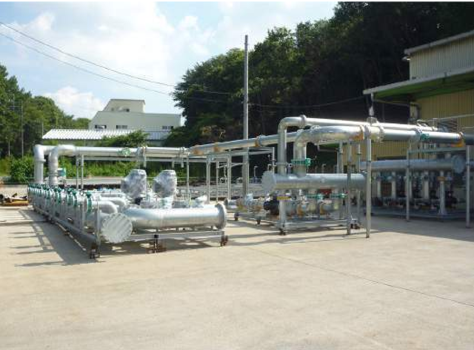
Figure 11: Prefabricated plant modules fitted and lined up in factory (Photograph courtesy of Seikei factory, Japan)
