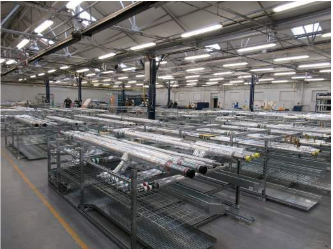
Figure 12: Alignment of modules in a factory. Prefabricated MEP modules are fitted out in the factory, prior to delivery and installation on site ( Photograph courtesy of DSG Modular )
