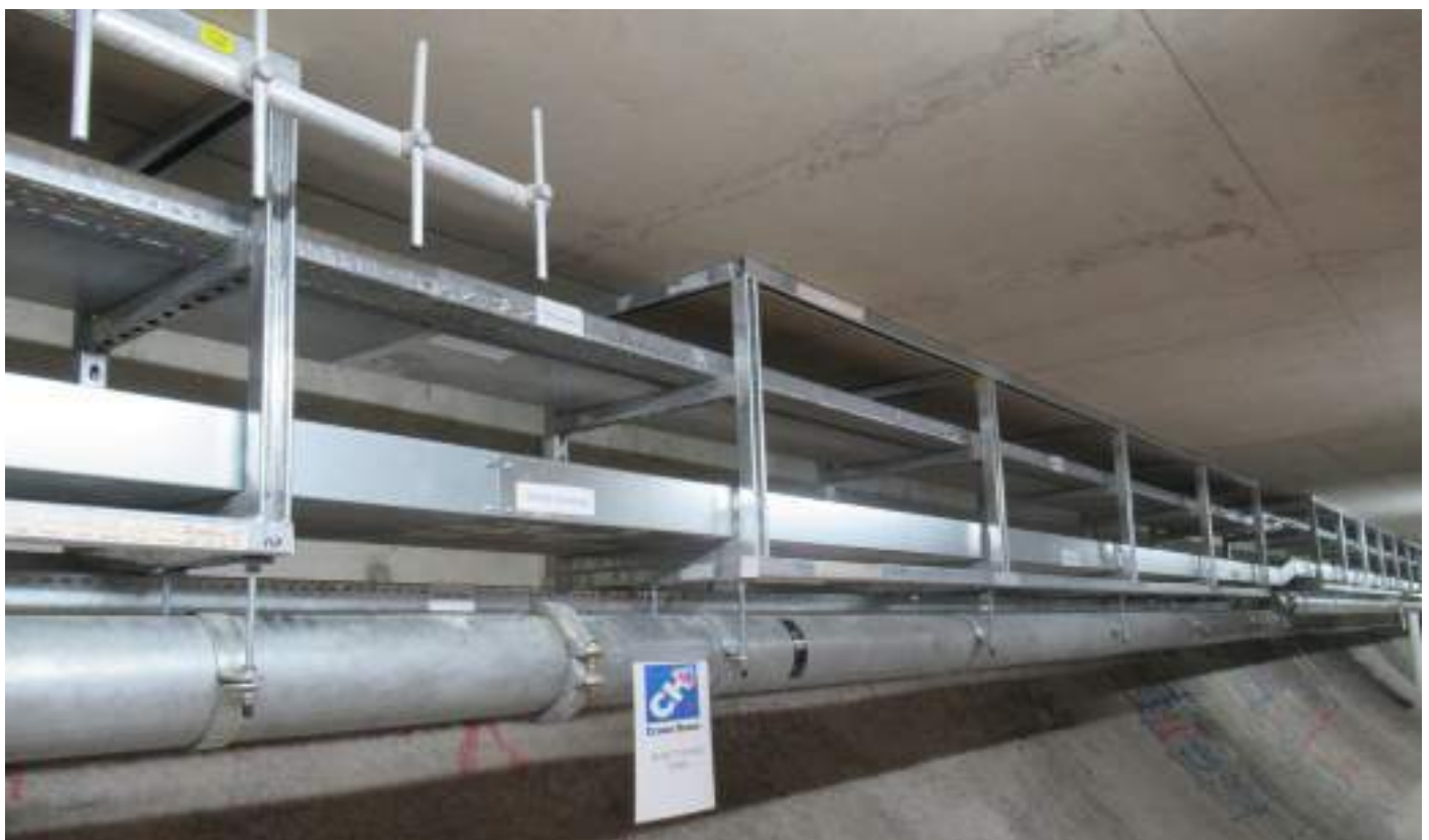
Figure 18 (Top): Prefabricated modules in the services tunnel. (Photograph courtesy of Laing O'Rourke)
